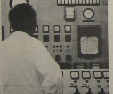
Power worker in the control room of Munroah Power Station, NSW.
