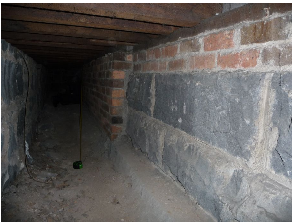
Under the GMT Chamber floor, looking south. The floor is supported by the bluestone wall at the left and by the bricks on and alongside the plinth on the right. The soil is remarkably dry.
