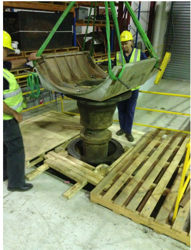
The Cradle is located and bolted on top of it. The telescope tube will sit in the Cradle, but not yet!
