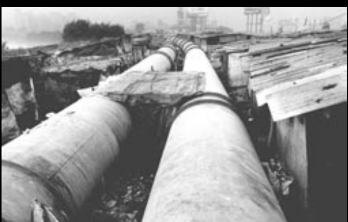
Water pipes, Bombay, India, 2001 - Paul Blackmore
