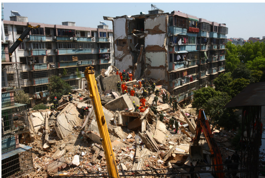
This building collapse in Fenghua city, Zhejiang province on April 4, 2014 buried 7 people, killing one. Inspectors warned the rest could also collapse. Photo: China Daily
