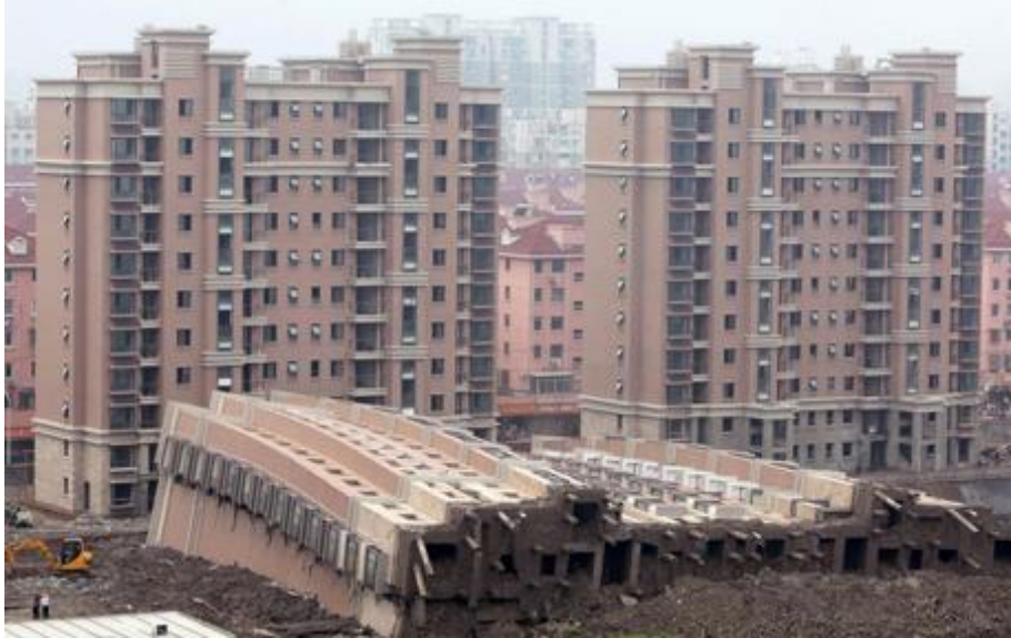
In June 2009, this nearly finished 13-story apartment building in Shanghai just toppled over killing a construction worker. Photo: Reuters
