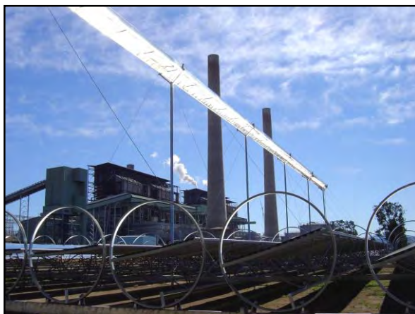
Figure 12: Concentrating linear Fresnel reflector at Liddell Power Station, NSW
