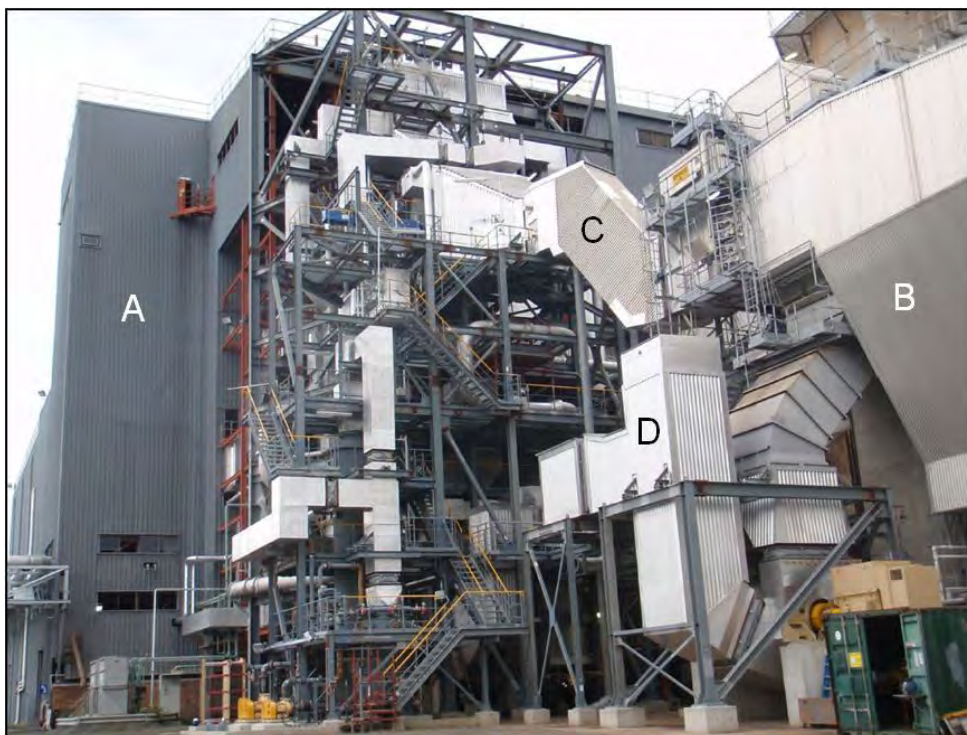
Figure 146: View of Callide oxyfuel boiler equipment
