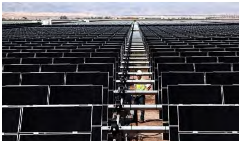
Figure 21: 250 MW Silver State solar project, which includes one of the world’s largest SAT systems
