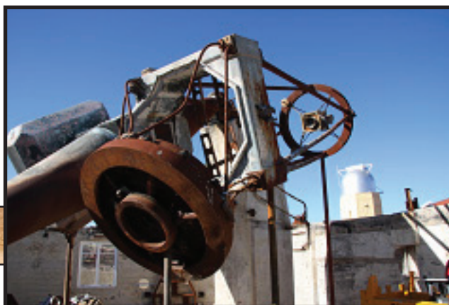
This photograph breaks my heart. The mirror cell is supposed to line up with the square holder and the top end.
