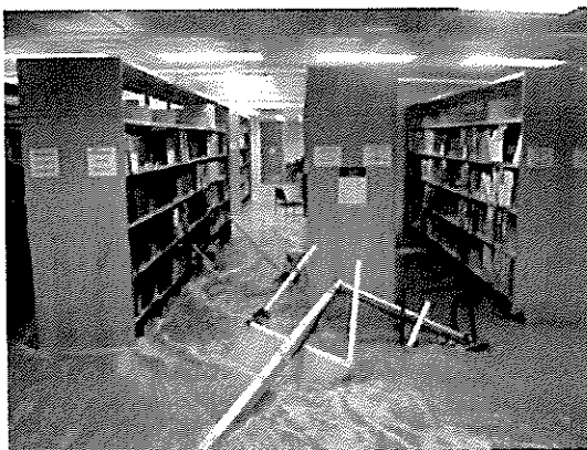
Figure 12: Photograph of major flash flood damage to a library in the University of Western Australia.
