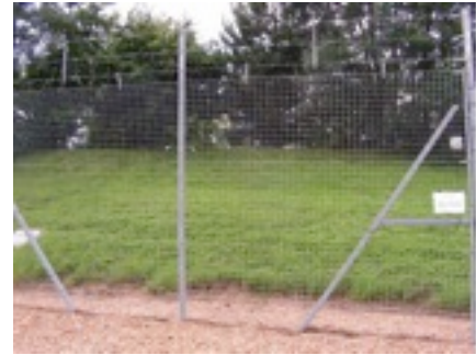
Picture 2: Class 2 security fencing
