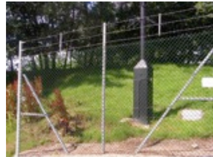
Picture 1: Class 1 security fencing
