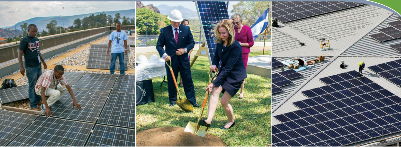
Images (Left) to (Right): (1) Local staff replace a photovoltaic module at the U.S. Embassy in Kigali, Rwanda; (2) Bobbie Griffin of Lockheed Martin, Donna McIntire of State's Bureau of Overseas Buildings Operations, and Ambassador Phyllis Powers break ground for the Energy Savings Performance Contract in Managua; and (3) A photovoltaic system is being installed on the roof of the parking garage at the U.S. Consulate General in Monterrey, Mexico, April 2015. State Magazine
