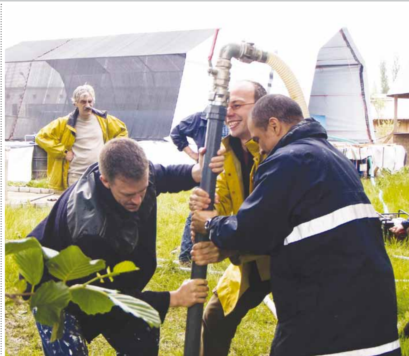
Constructing an emergency water borehole at Espace Bruno Corbé, the training facility for MSF field workers in Belgium Photographs: © MSF, 2010
