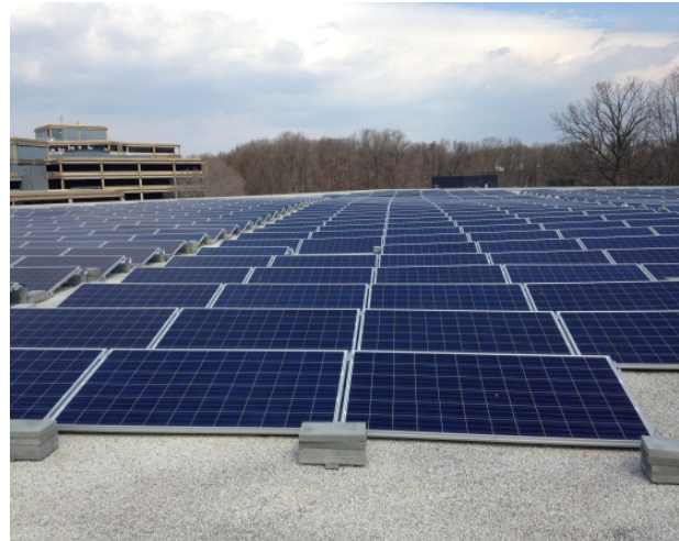
125 KiloWatts Photovoltaic (PV) Array Recently Installed at the USGS National Center, Reston, VA Photo by Calvin Graves, USGS
