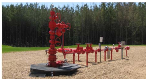
A carbon dioxide injection well in Mississippi.
