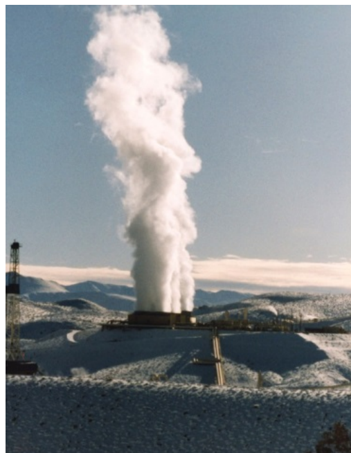
Figure 9: Coso geothermal plant, Navy One, at Naval Air Weapons Station-- China Lake in southern California.
