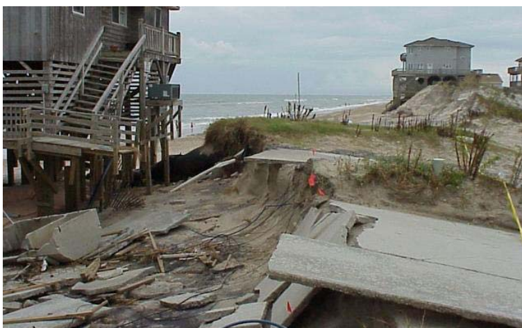
Figure 3: Parking areas, septic systems, and foundations in South Nags Head, North Carolina, collapsed when the underlying dune was eroded during the September 1999 landfall of Hurricane Dennis.
