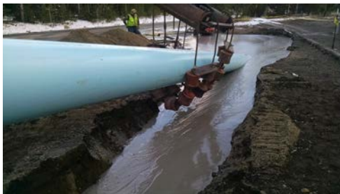
A section of new pipe is being monitored as it is placed (or replaced) as part of the Fishing Bridge Waterline rehabilitation
