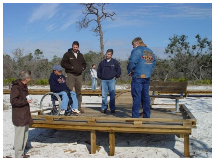
Visitor Facility Enhancements such as this accessible observation deck at Bon Secour NWR (AL) allow all visitors to get out on the land to experience refuges first-hand. Photo credit: Steve Hillebrand
