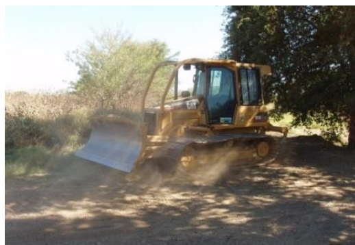
Heavy equipment enables the Service to accomplish habitat management, refuge operations, and visitor services goals.
