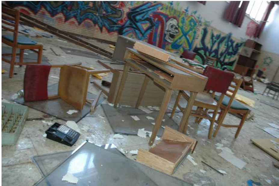
After Attucks Elementary students and staff were removed from their building at 39th and Dearborn into a new building, CPS failed to secure the facility. Today it is filled with trash, gang graffiti and empty beer cans. Closing these schools does not save resources, it wastes them. Photo: Nathan Goldbaum
