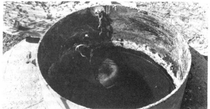
Float-valve regulates water level in stock tank.
