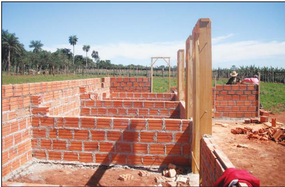
Picture 23: Cooperative farmers in Paraguay are building this fertilizer and chemical storage shed. Built under the strict specifications of GLOBALGAP, the chemicals applied to the crops can be handled in a professional manner.
