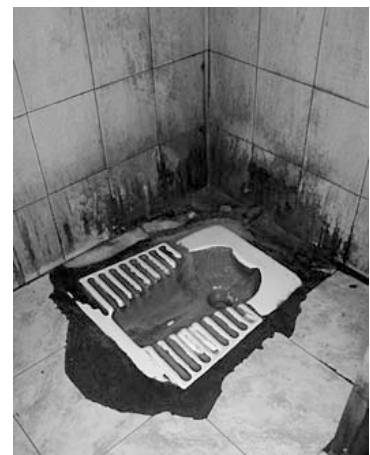
Toilettes in detention are usually not working or/ and very dirty
