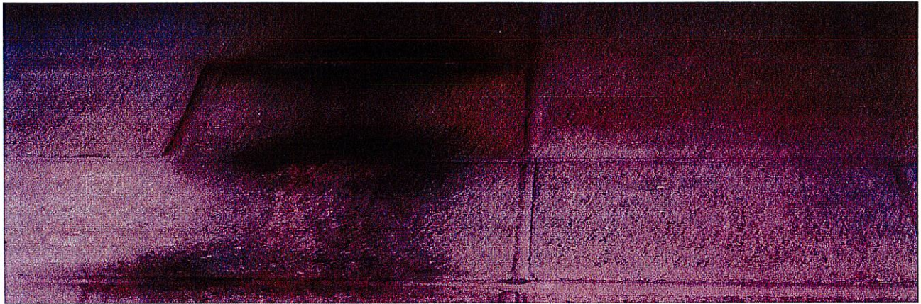
Picture 2: Water stain-moving up along the cinder block from the cooling and ventilation units
