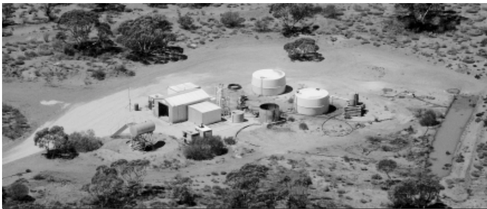
Figure 6.28 Village reverse osmosis water plant—supplies fresh water to Maralinga village.
