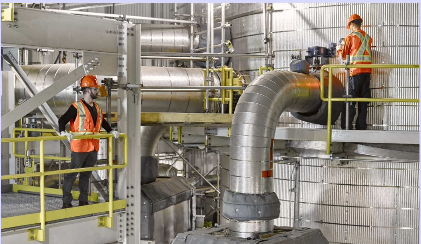
Carbon capture infrastructure at the Boundary Dam. SaskPower
