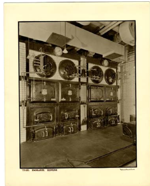
The state-of-the-art boilers in the basement. Courtesy Museum of the City of New York.
