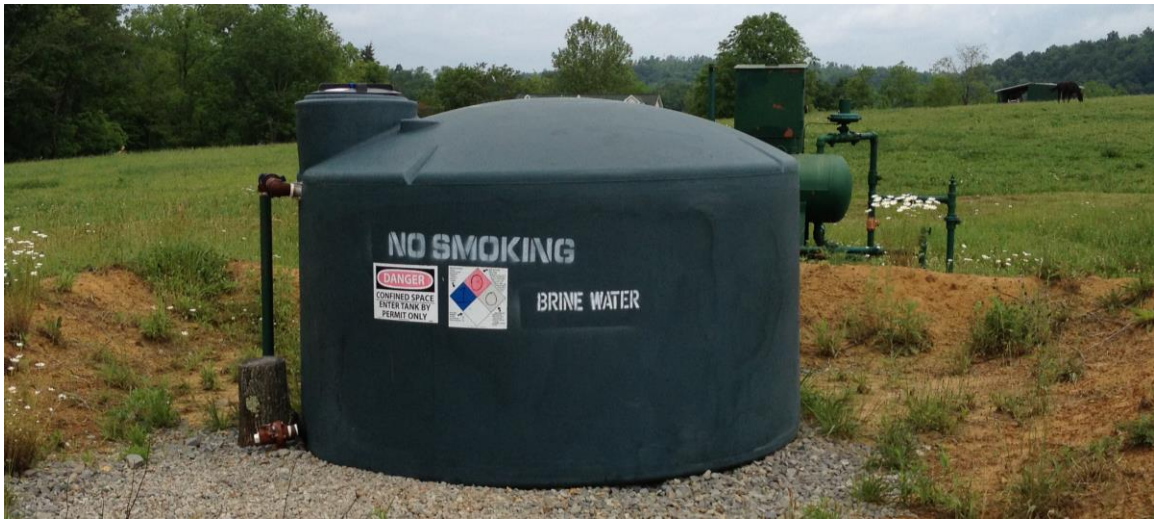
Brine storage tank. Photo by Nadia Steinzor.
