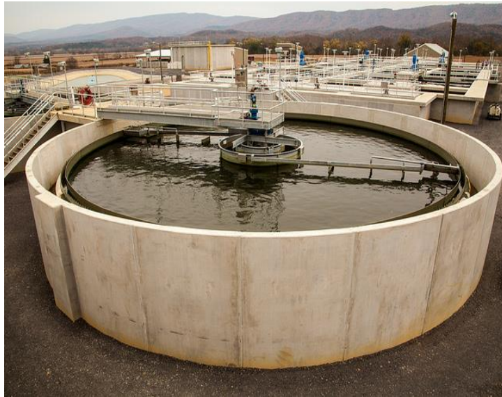
Wastewater treatment plant in West Virginia. Photo courtesy of Chesapeake Bay Program.
