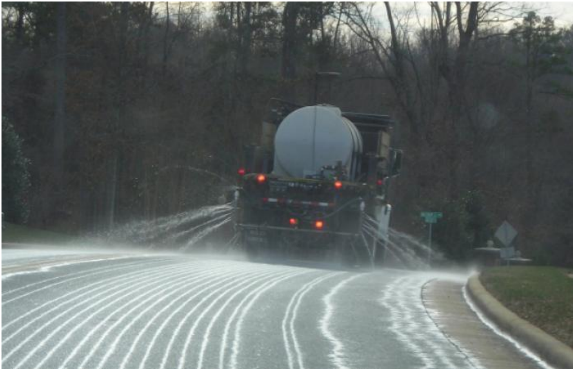
Truck spreading brine in New York. Photo courtesy of No Fracking Way.
