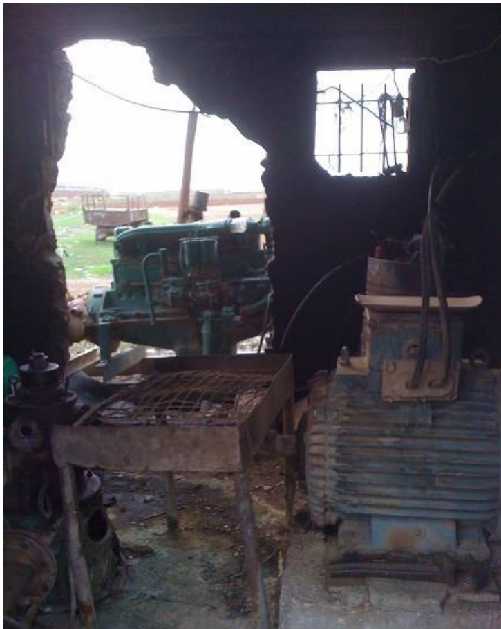
Well house at Deir Ghazaleh
