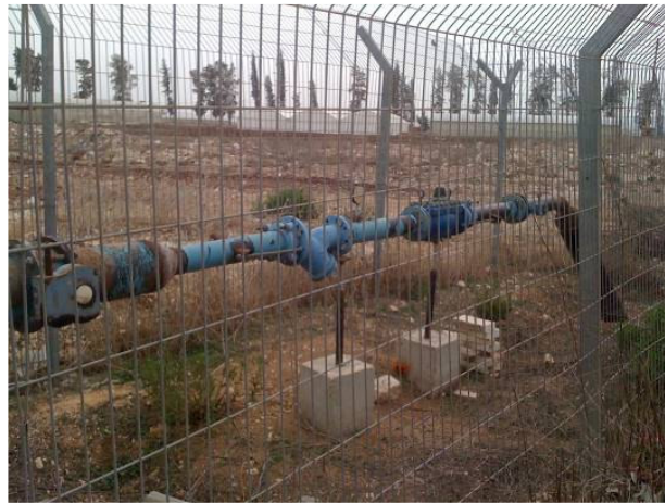
Mekorot line in Jalama.
