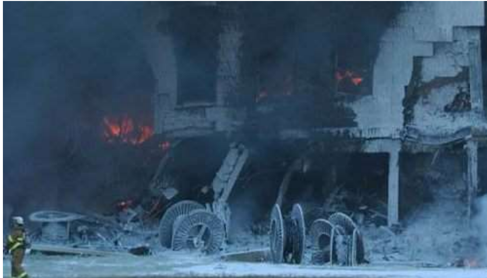
Figure F-14 Façade damage with some fire Taken at a less oblique angle facing the façade
