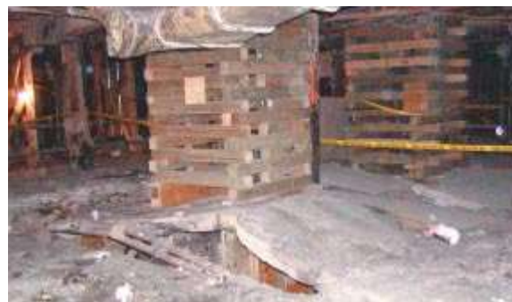
Figure H-2 Pentagon Building and Performance Report Figure 5.27 Breached second-floor slab
