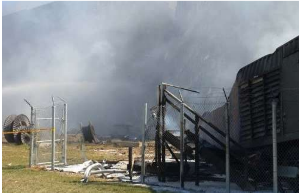
Figure F-4 Generator trailer and fence The north end of the trailer is gouged
