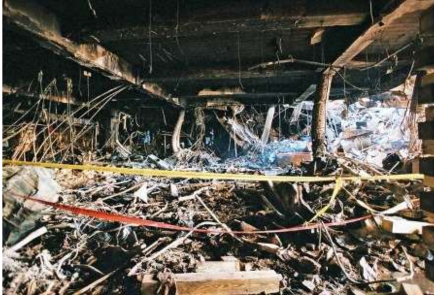
Figure G-3 Internal debris and curved columns
