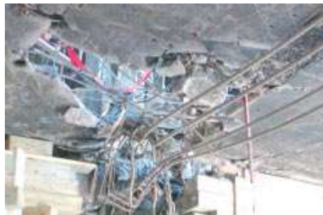
Figure H-3 Pentagon Building and Performance Report Figure 5.29 Stripped floor beams under second-floor slab
