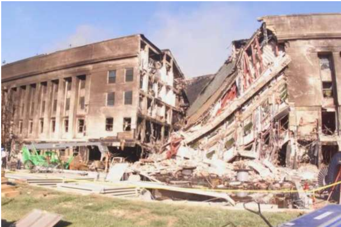
Figure F-8 Warning lights and collapsed section (see red lights at bottom right)
