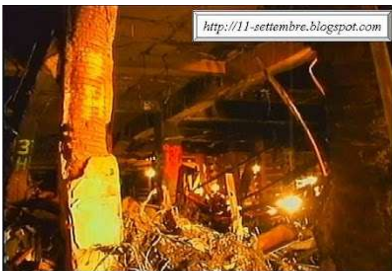
Figure G-1 Curved and abraded column
