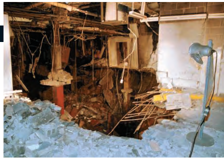
Bomb damage at the WTC
