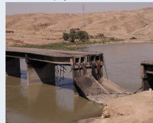
Coalition bombing damaged al-Fatah Bridge in 2003.
