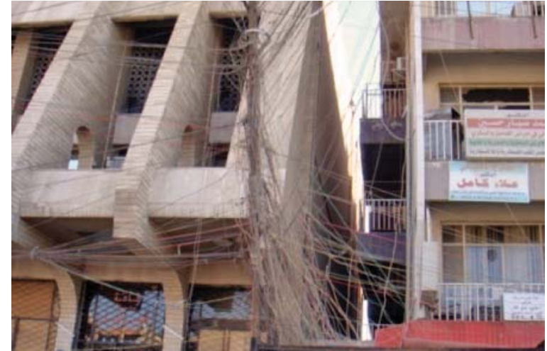
A tangle of consumer-installed electric wires carries power from private generators to households in central Baghdad. (Parsons Brinckerhoff photo)
