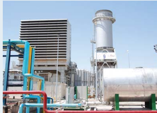
The United States spent more than $250 million restoring the Qudas Power Plant under several different projects. (USACE photo)
