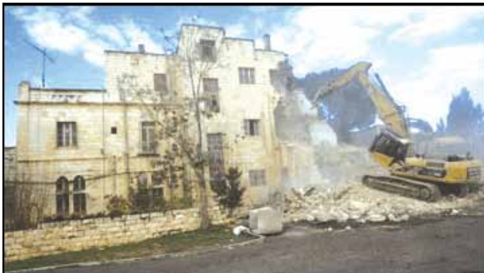
Photo: demolition of the “Shepherd Hotel”, January 2011. The hotel was declared “absentee property” and then sold to settler patron, Dr. Irving Moskowitz, who intends to build a new Israeli settlement on the property. (Photo by: Ahmad Gharabli/AFP/Getty Images).
