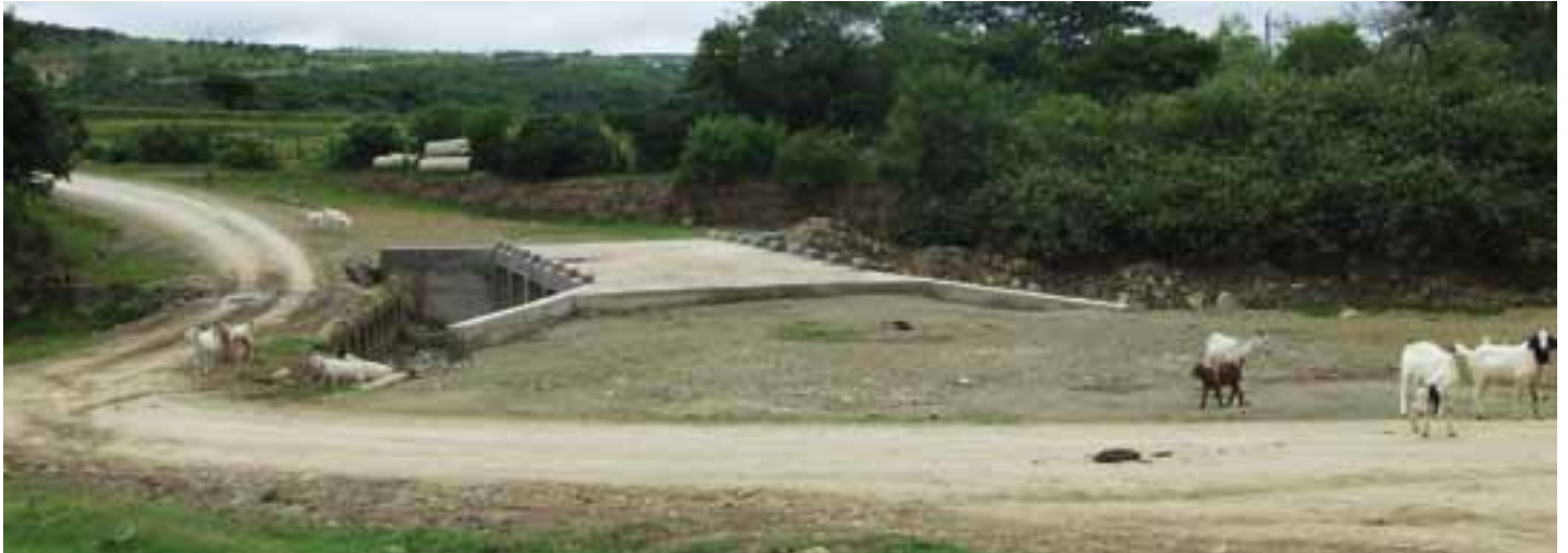
Lots of goats and a little white elephant: Mangqukela's bridge and the road passing nearby.
