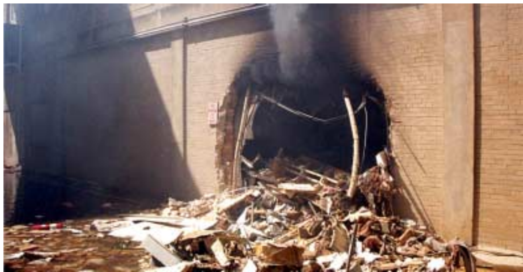
Penetration through the inner wall of the Pentagon's C Ring.
