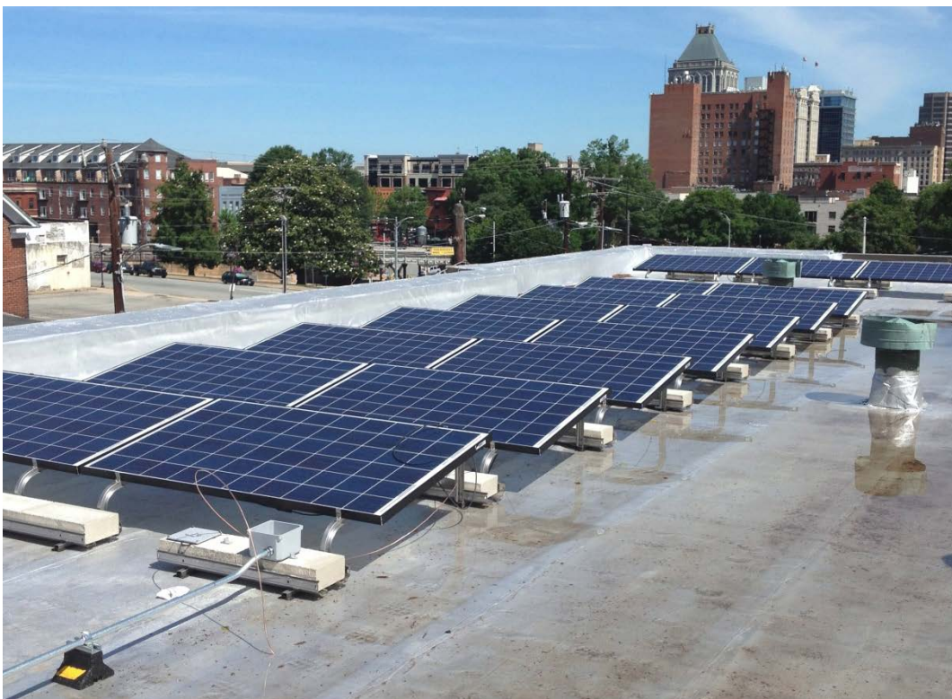
5 kW solar photovoltaic installed on the rooftop of Faith Community Church, 417 Arlington Street, Greensboro, NC 27406
