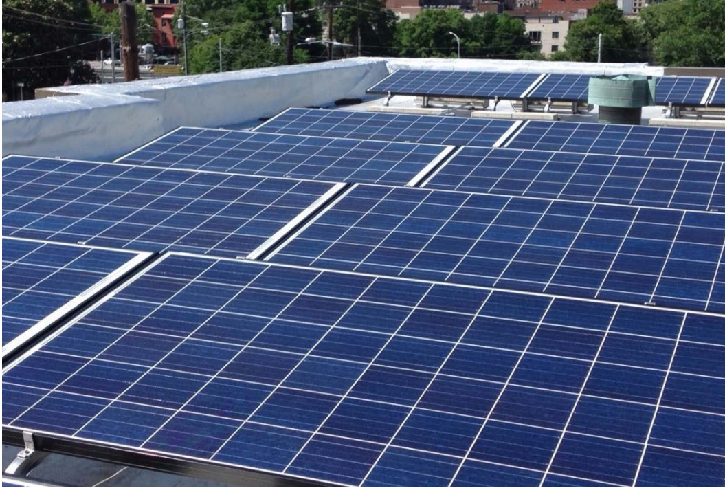
5 kW solar photovoltaic installed on the rooftop of Faith Community Church, 417 Arlington Street, Greensboro, NC 27406
