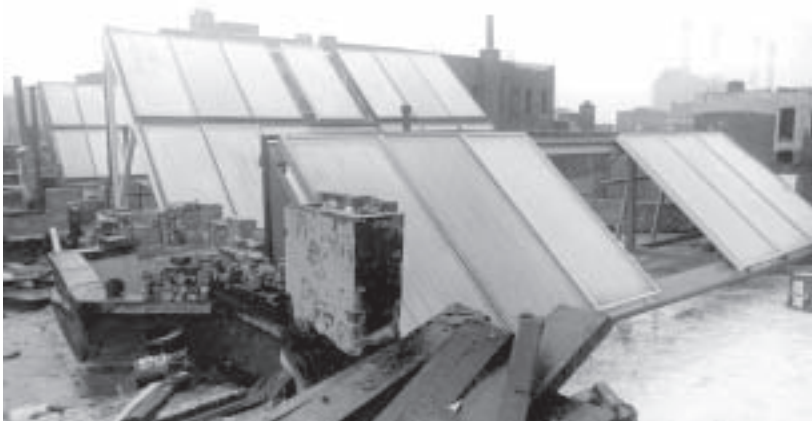
Solar Collectors on 519 E. 11 th St. NYC - 1976
