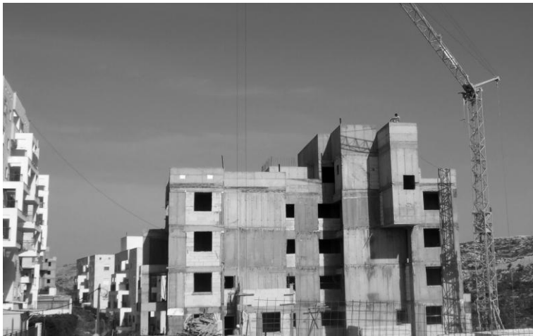
Building continues in the West Bank settlement of Mod'in Illit despite the construction ban (Corporate Watch 2010)
