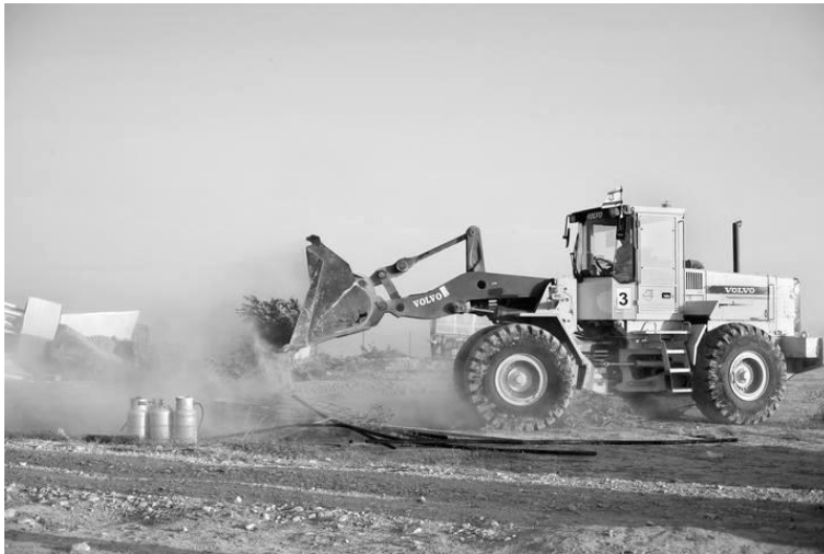
A Volvo bulldozer demolishes a structure in the Bedouin village of al-Araqib (Active Stills)
