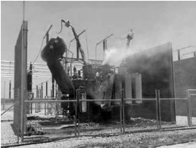
Gaza Power Plant after Israel bombed it with F-16s (International Solidarity Movement 2006)
