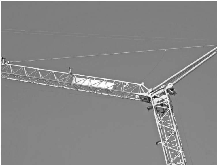
Crane looming over the ever expanding settlement of Mod'in Illit, Mod'in Illit is built on the land of the Palestinian village of Bil'in (Corporate Watch 2010)
