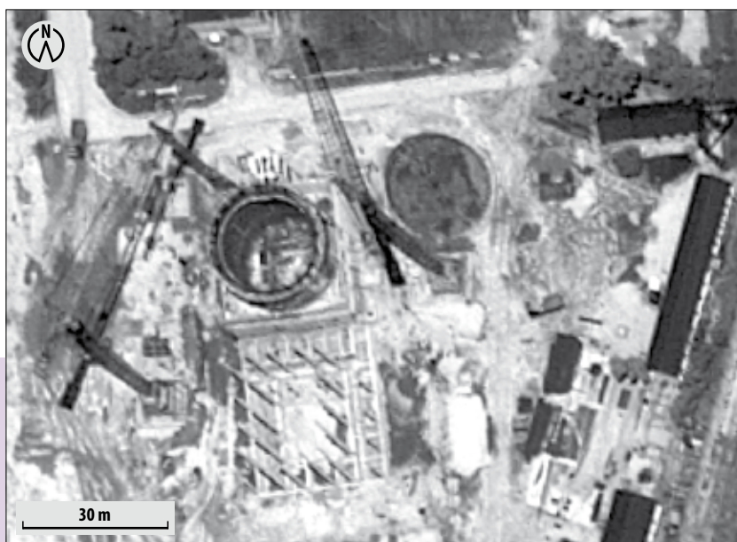
Construction site of the new reactor at the Yongbyon nuclear complex, North Korea [Geo-Eye; photo dated 5 September 2011]
