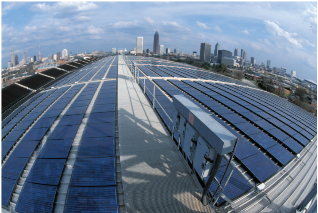
Commercial-scale rooftop solar PV array.
