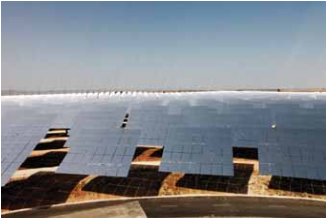
Above: Heliostat mirrors, Torresol Gemasolar power plant, Spain. Image courtesy Markel Rodondo
