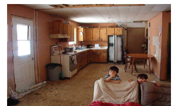
Inside a home at Rapid Lake needing repairs.
