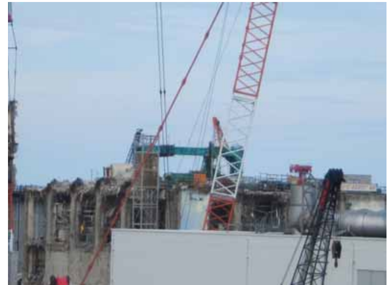
-3 Appearance of Unit 4 (View from the southern hill) Photo taken by a TEPCO employee on September 5, 2012
