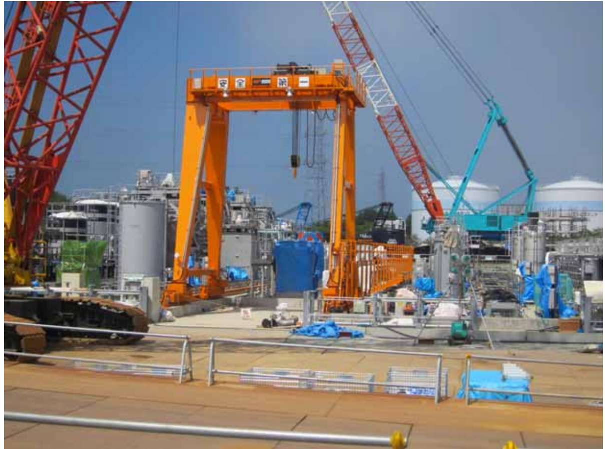
-2 Multi-nuclide Removal Equipment construction site: Installing equipments, etc. Photo taken by a TEPCO employee on August 21, 2012
