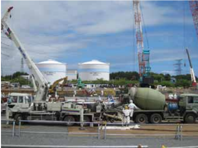
-1 Multi-nuclide Removal Equipment construction site: Foundation improvement work Photo taken by a TEPCO employee on June 11, 2012
