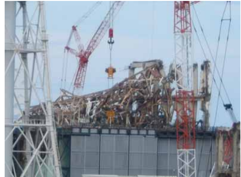
-2 Appearance of Unit 3 (View from the southern hill) Photo taken by a TEPCO employee on September 5, 2012
