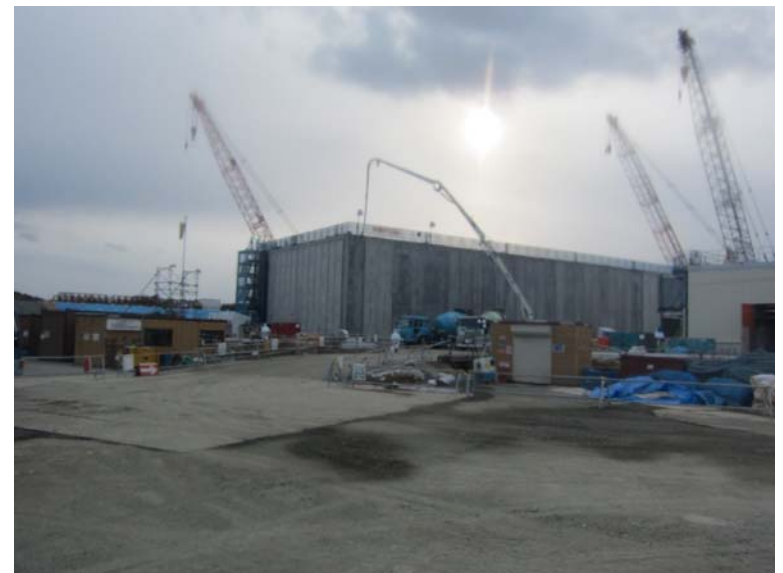
⑥-3 Waste sludge storage facility Jan. 9, 2012 photo by TEPCO staff
