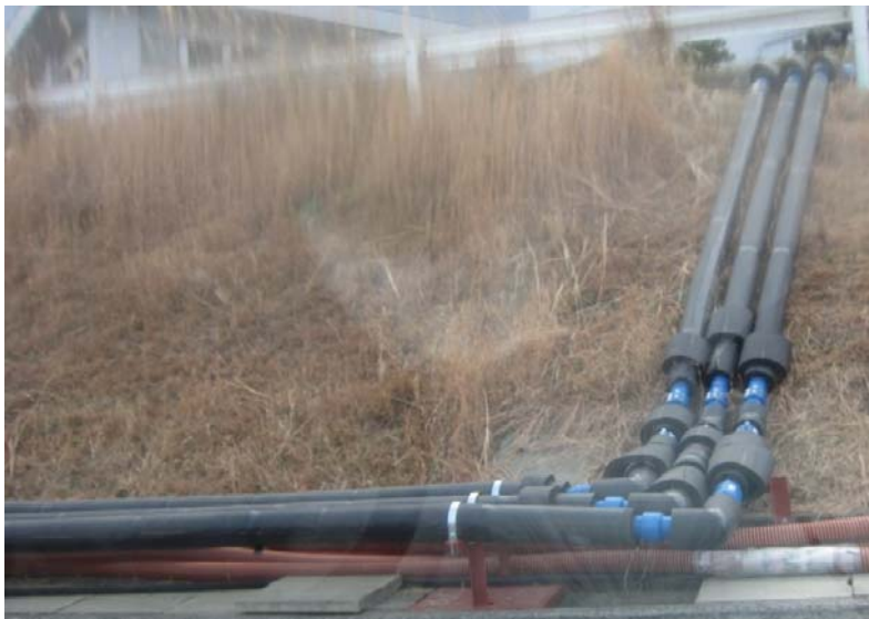
⑨ Anti-freezing measure for the reactor injection hose Jan. 9, 2012 photo by TEPCO staff
