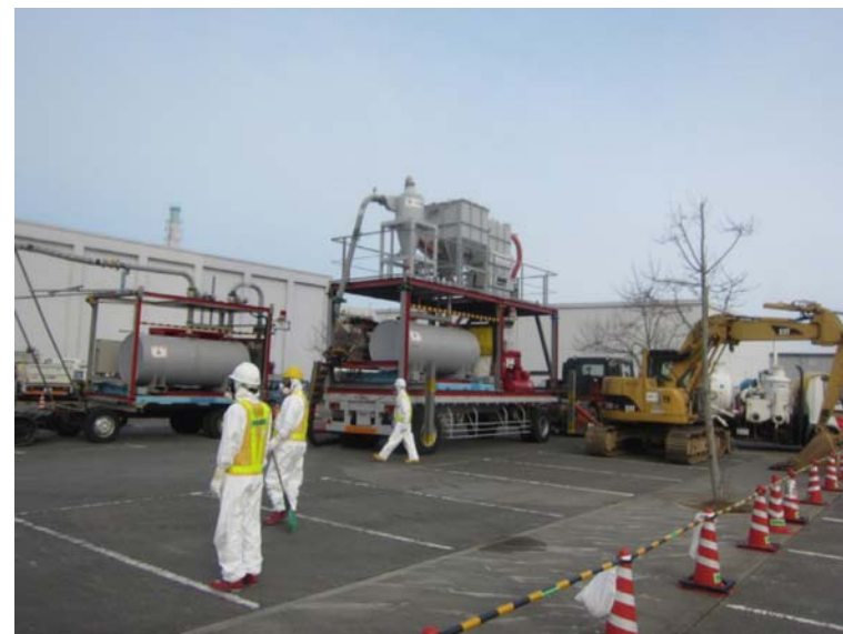
②-2 Collection work of dust and small debris at parking area of Main Anti-earthquake Building
