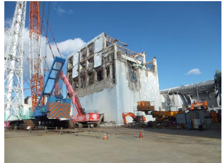
①-8 Removal of debris on the upper side of Unit 4 Reactor Building (after work)
