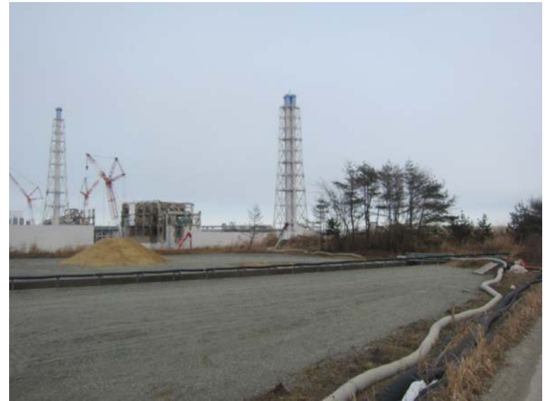
④-2 Look into Reactor Building from the hill in the southern side of Unit 4 Jan. 9, 2012 photo by TEPCO staff
