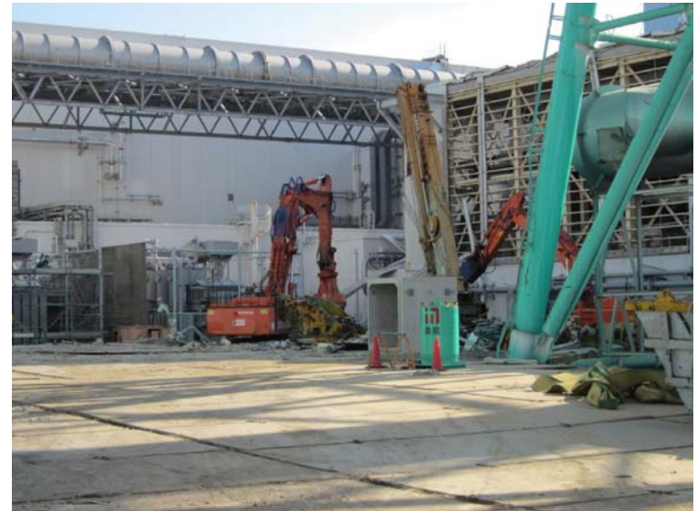
①-2 Removal of debris around Unit 3,4 Reactor Building Jan.10, 2012 photo by TEPCO staff
