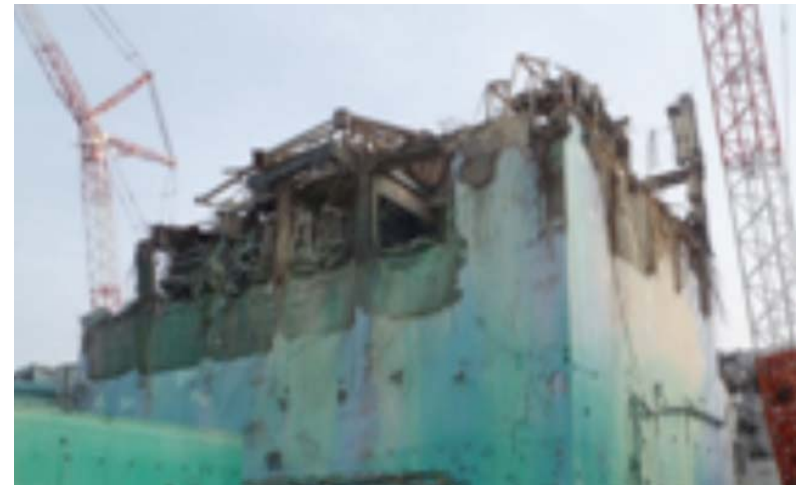
①-6 Removal of debris on the upper side of Unit 3 Reactor Building (after work)
