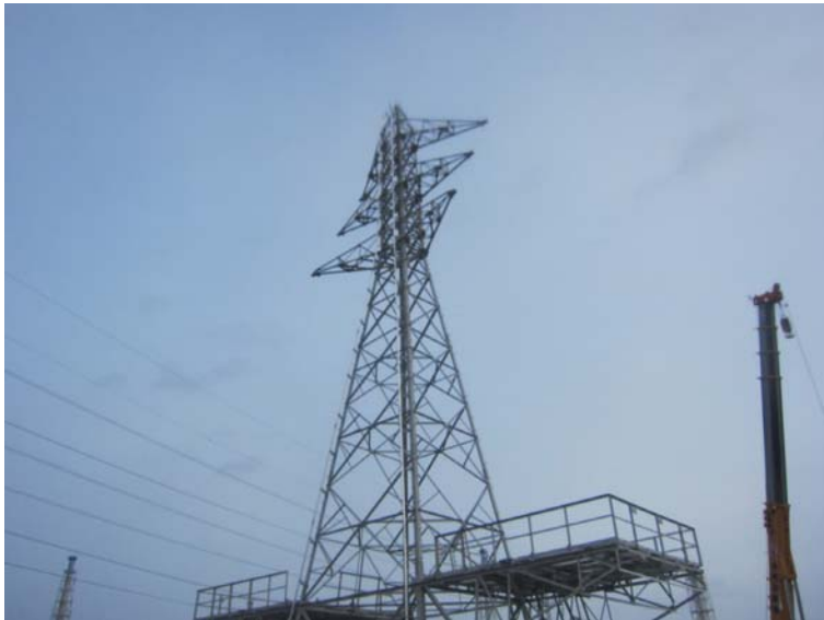
⑦-1 Lead-in tower from new switch station Jan. 9, 2012 photo by TEPCO staff
