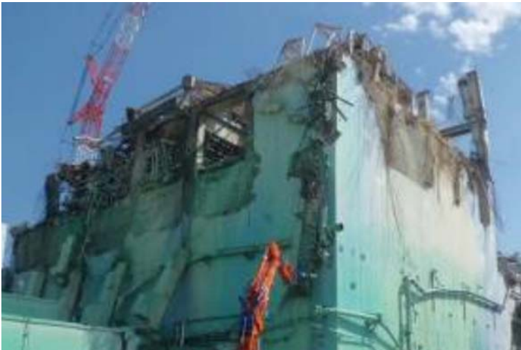
①-5 Removal of debris on the upper side of Unit 3 Reactor Building (before work)
