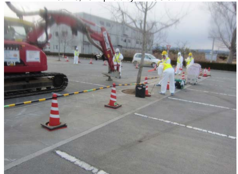
②—6 Collection work of dust and small debris at parking area of Main Anti-earthquake Building
