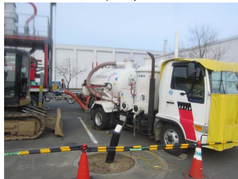
②-3 Collection work of dust and small debris at parking area of Main Anti-earthquake Building
