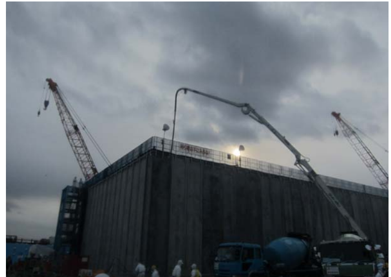
⑥-1 Waste sludge storage facility Jan. 9, 2012 photo by TEPCO staff
