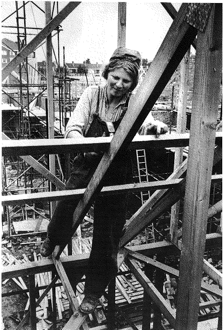
Sue Shearer, a member of 'Women in Manual Trades', on a building site at the Elephant & Castle, London, where she works as a carpenter (Carlos Augusto, IFL)
