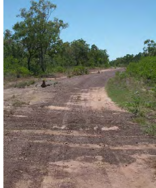
PHOTOGRAPH G3.21 Access road through site – view 2 showing erosion damage
