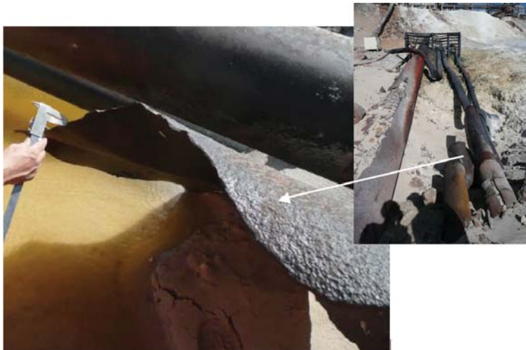
Photo 14 – Ruptured section 12" sales gas line, external corrosion and wall thinning
