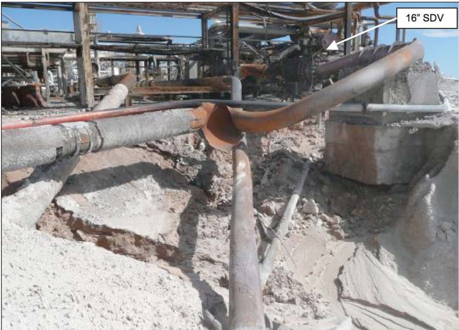
Photo 10 – Ruptured 16” sales gas line
