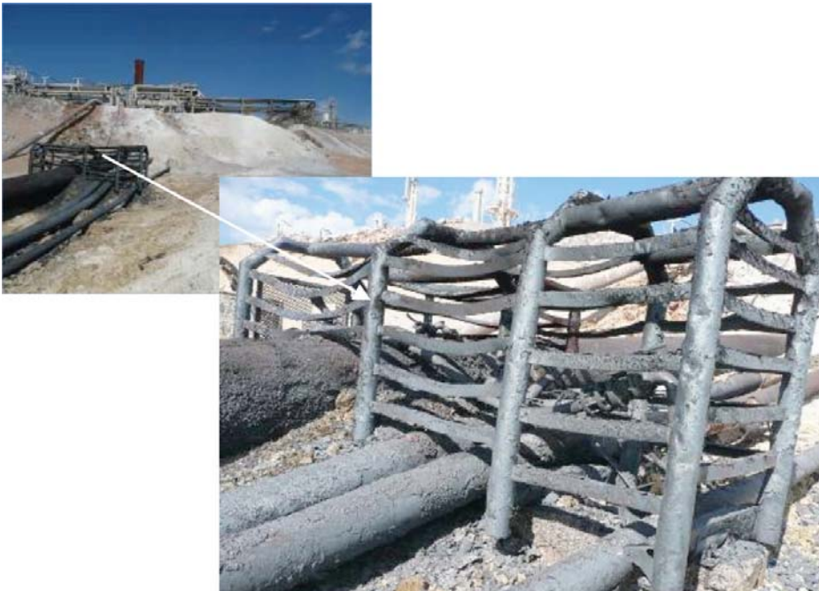
Photo 6 – 30” crude export line valve cyclone protection cage
