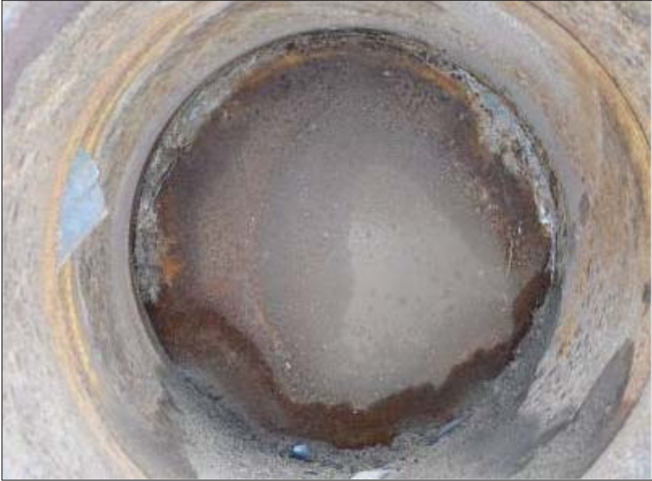
Photo 16 – Inside view of 16” SDV, ball in closed position
