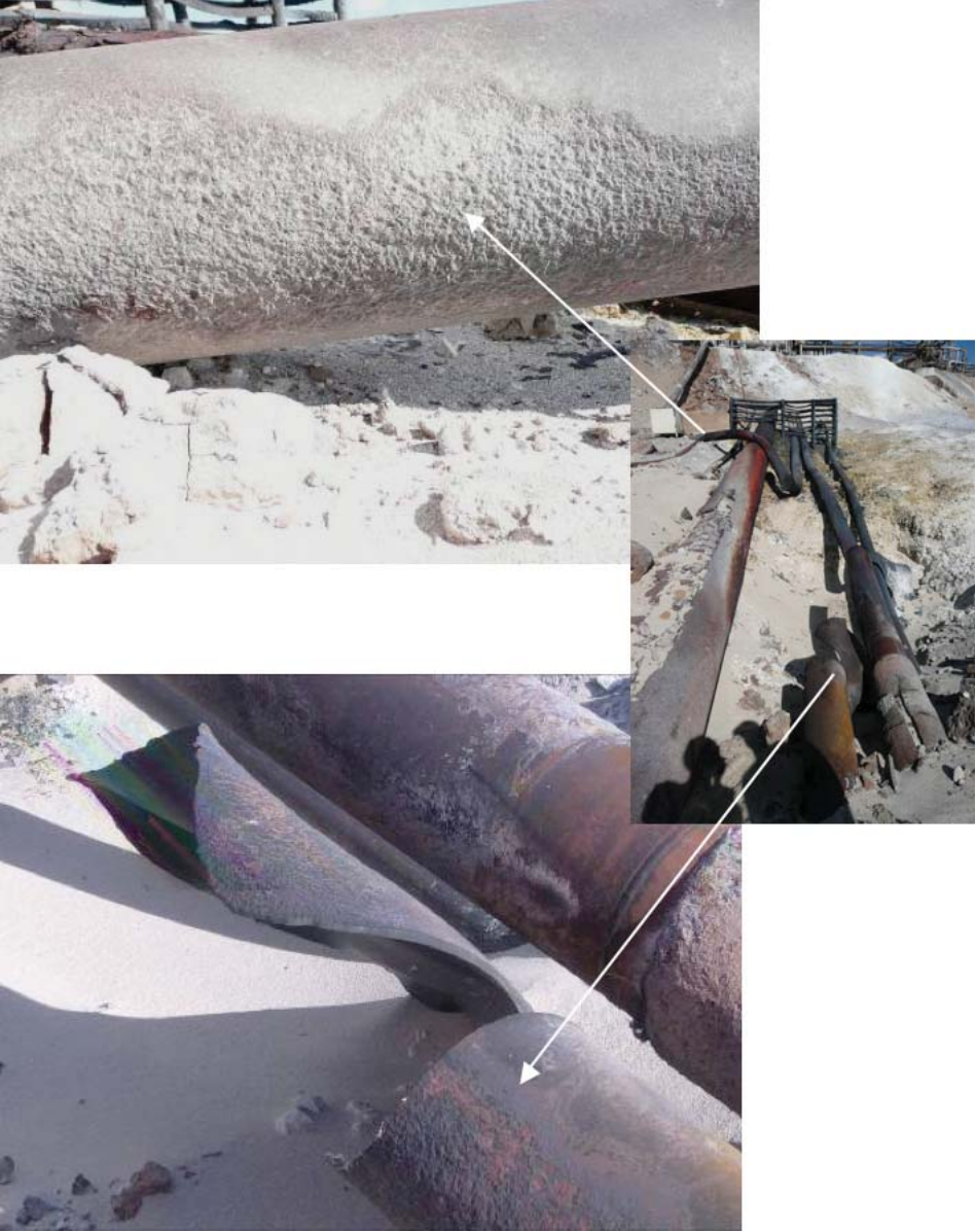
Photo 15 - Ruptured section 12" sales gas line external corrosion
