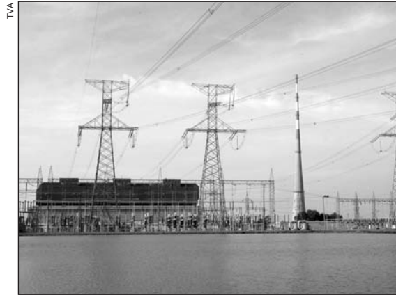
BROWN'S FERRY —In 1975, a worker using a candle to check for air leaks, started a fire that closed the Brown's Ferry nuclear plant for two decades. In 2011, a tornado cut power to the rebuilt reactors, triggering an emergency shutdown.
