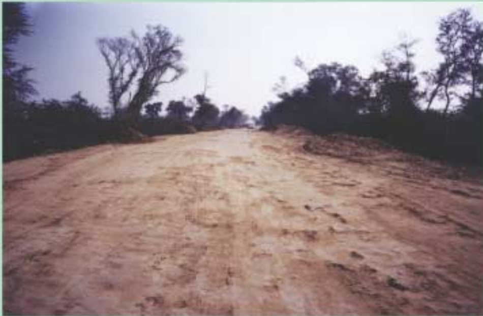
A stretch of the National Highway No. 10 between Mandi Dabwali, Haryana and Malout, Dist Muktasar, Punjab. The road is being raised and repaired as it has suffered extensive damage due to waterlogging.
