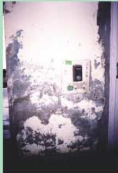
Dampness along the wall at a house in Malout town, District Muktsar, Punjab leading to peeling off of the paint and plaster. Waterlogging has impacted about 70% of the houses in this town, and houses require repair at regular intervals.
