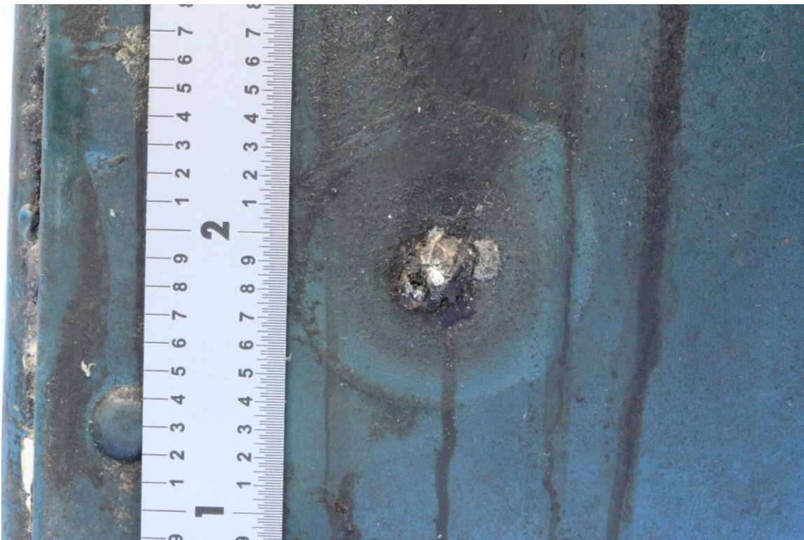
Figure 14. Protrusion on the lower left of battery cases side 3.
