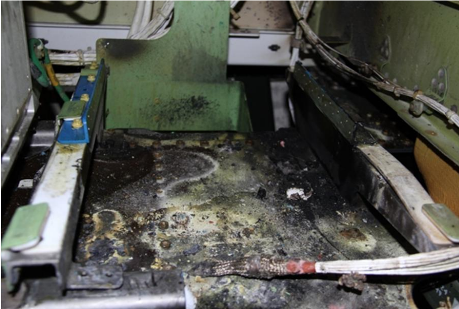
Figure 5. Auxiliary power unit installation location with battery removed.
