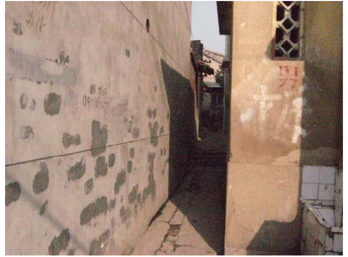
Inside the South Wall: Substandard Housing 158
