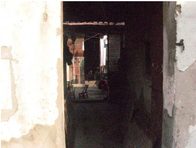
Inside the South Wall: Substandard Housing 165
