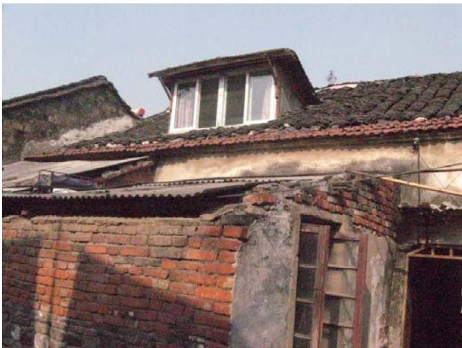
Inside the South Wall: Substandard Housing
