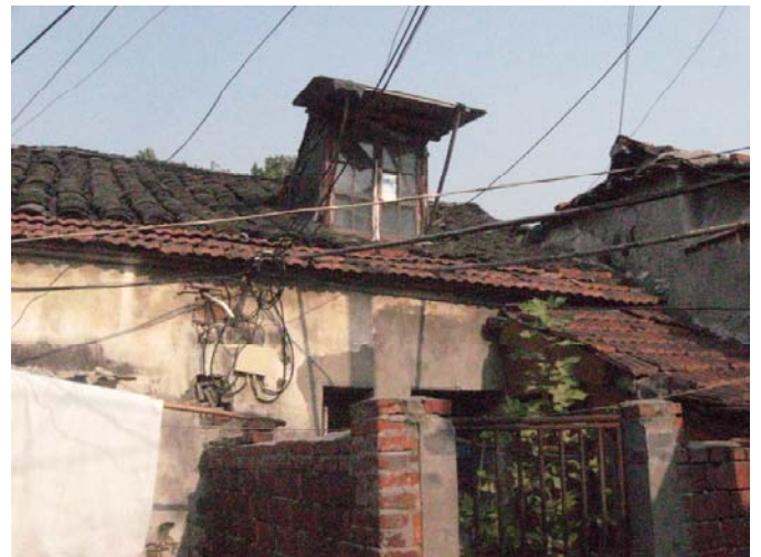
Inside the South Wall: Substandard Housing
