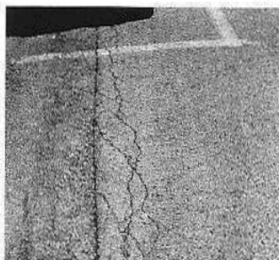
.b. Medium-severity edge cracking
