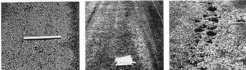
.a. Low severity weathering and raveling
