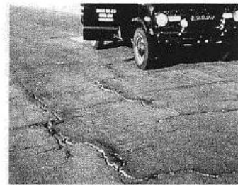
High Severity block cracking
