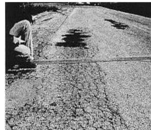
c. High-severity alligator cracking
