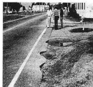
.c. High-severity edge cracking
