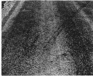
.a. Low-severity bleeding
