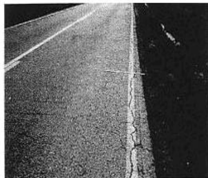
b. Medium-severity alligator cracking
