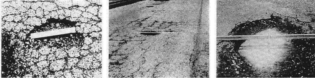
.a. Low-severity pothole .b. Medium-severity pothole .c. High-severity pothole
