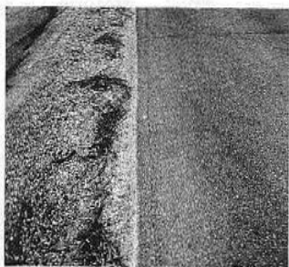
.a. Low-severity edge cracking
