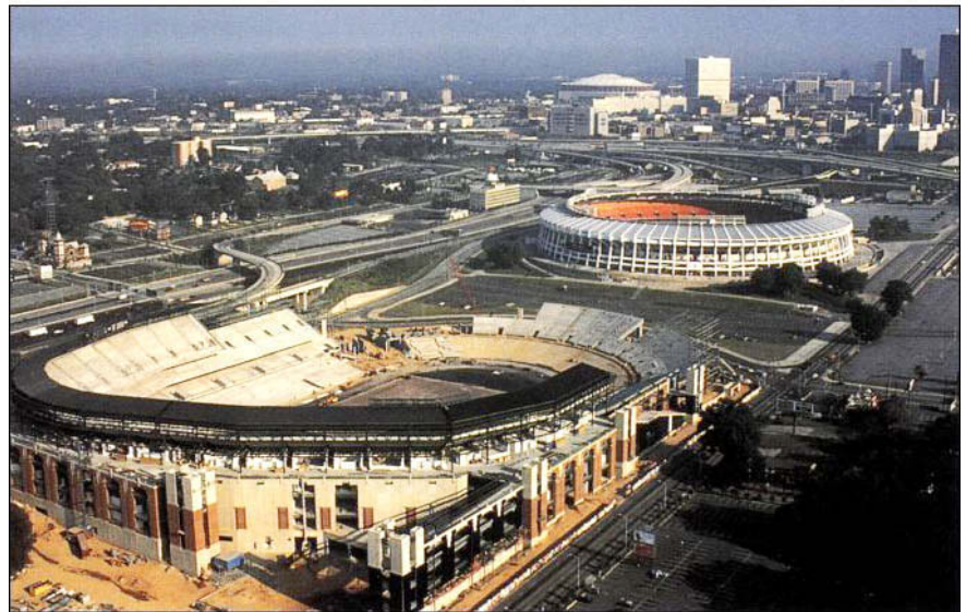
These two views show the Olympic Stadium site when construction had just begun ( top ) and when work was nearly complete ( bottom ).
