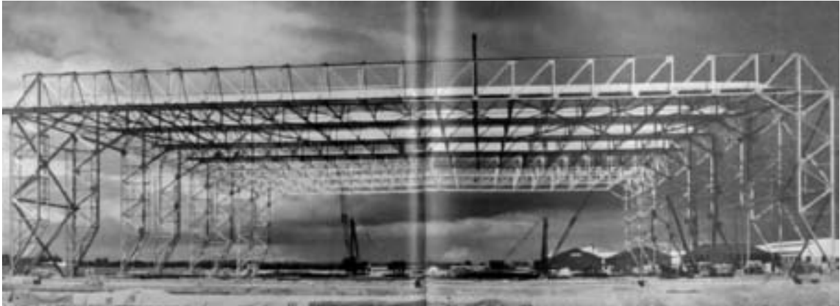
Fig. 39: De Havilland Avion Hanger, trussed aluminum frame structure spanning 61 m. James M. Monro & Son, 1955. (Peter)
