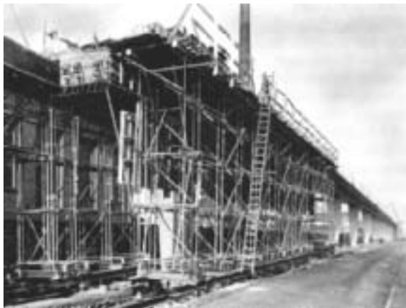
Fig. 47: Rail mounted formwork used for a pedestrian and bicycle bridge at the Casellastrasse in Frankfurt/Main, Germany. (Wittfoht)
