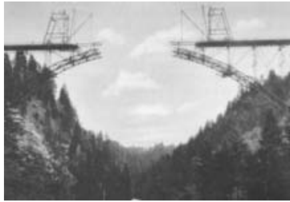
Fig. 37: Erection of the steel lattice truss to construct the Ammer Bridge at Echelsbach, Germany, using the Melan Method, 1929. (Wittfoht)
