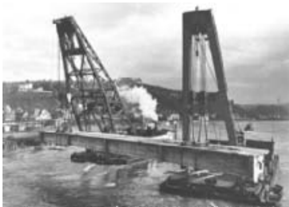
Fig. 39: 150 metric ton precast, Prestressed concrete girder being floated into position by enormous cranes for the bridge over the Rhine at Vallendar, Germany, 1959. (Wittfoht)
