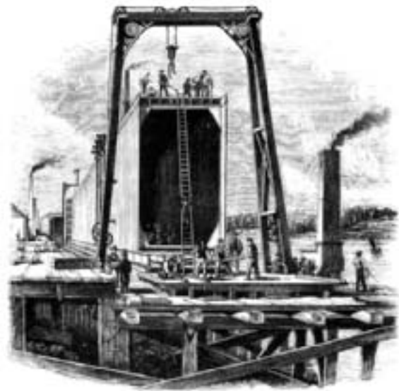
Fig. 67: Britannia tubes under construction on assembly platform with mobile gantry cranes. (Peters 1 )
