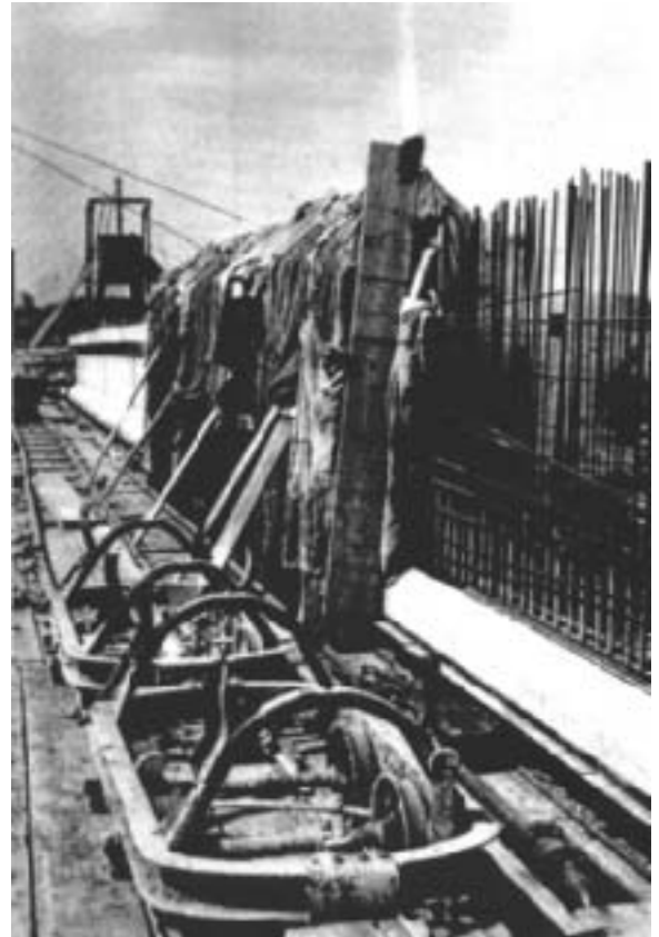
Fig. 22: Fabrication of the pre-cast prestressed concrete girders for the Ölde Bridge. The rear section of the girder is complete; the central section is hooded for steam heating; and on the right, only the lower flange has been cast. (Grote and Marrey)
