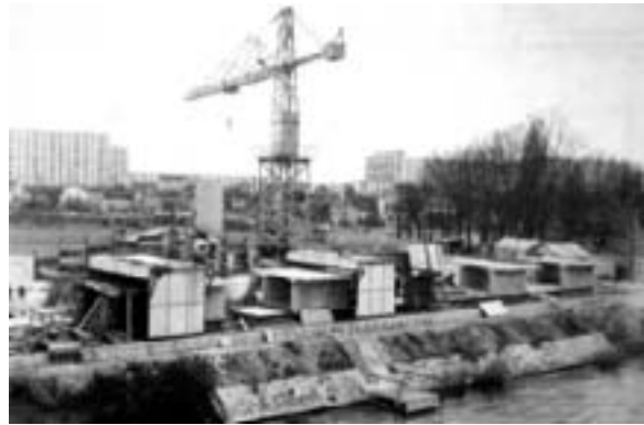
Fig. 56: Match-cast box girder segments in precasting yard for the construction of the Choisy-le-Roi Bridge, France. (Podolny and Muller)
