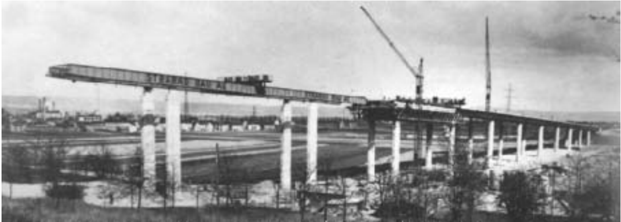
Fig. 48: Bridge on the Kettinger Hang for the B 9 between Bonn and Koblenz, Germany, first prestressed concrete bridge built using self-supporting traveling formwork, 1959. (Wittfoht)
