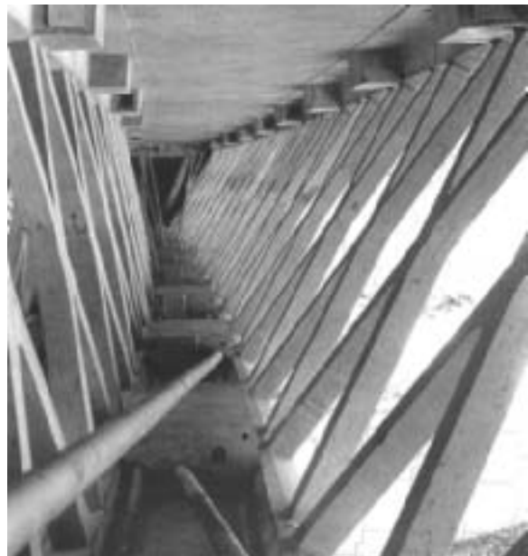
Fig. 72: Box section with lattice-type webs and external prestressing. Glacières Viaduct, France. (Marrey)
