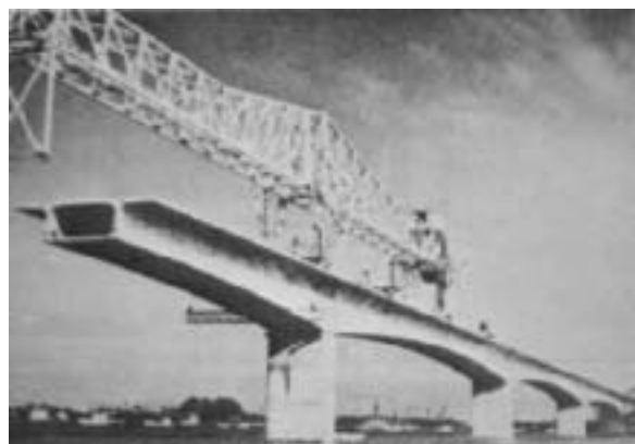
Fig. 58: Oleron Viaduct, construction view showing cantilever span. (Podolny and Muller, after the American Concrete Institute)
