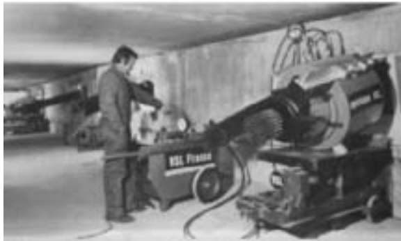
Fig. 79: (a) Diagram showing access hole provided for tensioning jack. (b) View of jacking procedure. (SETRA)
