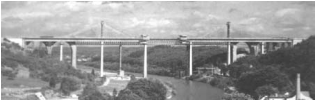
Fig. 45: Example of cantilever construction method using auxiliary cable stays. Image shows construction of the Lahntal Bridge at Limburg, Germany. The bridge was commenced at both abutments and advanced toward the center. (Wittfoht)
