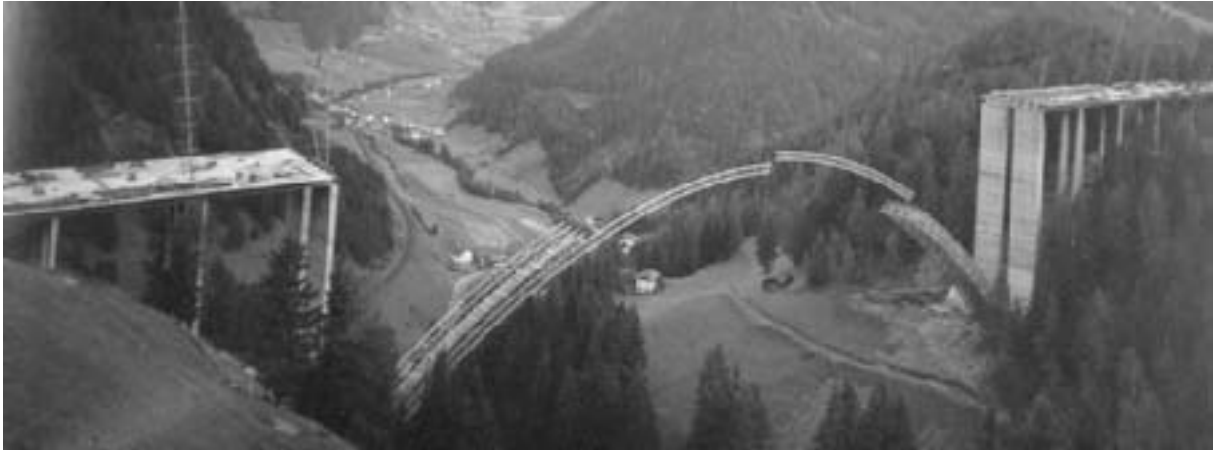
Fig. 38: Erection of the timber lattice truss centering with a 180 m span for the First Nösslach Bridge, Austria. (Wittfoht)
