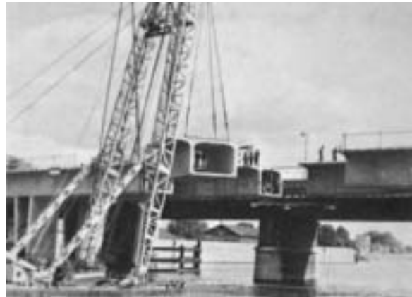
Fig. 57: Segment of the Choisy-le-Roi bridge being placed with a floating crane. (Podolny and Muller)
