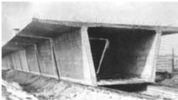
Fig. 54: Precast segments atop the guide-way used to construct the Ager Bridge in Austria, 1959-1962. Exposed rebar used to make mechanical connection with normal reinforcement between segments and to 50 cm gap left between segments used to facilitate tendon placement, after which the gaps were filled with concrete. (Wittfoht)
