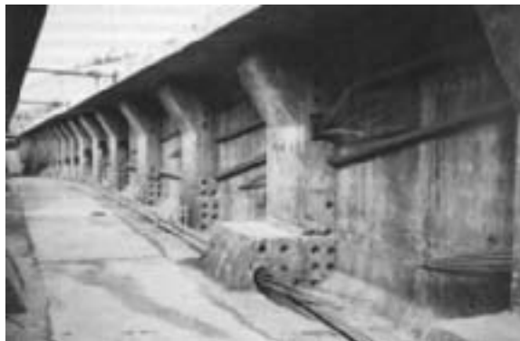
Fig. 74: Viaduct of Sermeaz, showing vertical arrangement of cables similar to geometry of Long Key Bridge without the same extreme eccentricities. (SETRA, after M. Virlogeux)
