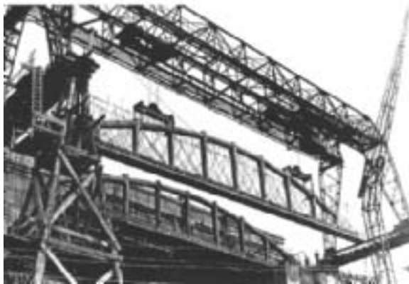
Fig. 24: Prestressed concrete roof girder with 30 m spans used to construct German submarine pen, 1943. (a) Cross-section of submarine pen. (b) Roof girder being lifted into place during construction. (Grote and Marrey)
