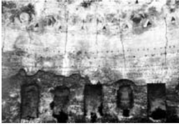
Fig. 28: (a) Cracking around the base of a concrete semi-dome, Baths of Trajan, Rome. (Mainstone 1 )
