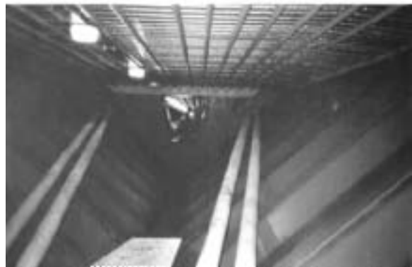
Fig. 71: Triangular section with closed webs of corrugated steel. Vallon de Maupré Viaduct at Charolles. (a) General view. (b) Inside triangular box girder. (SETRA)
