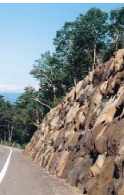
Rocks dug up on site during road construction were used for reinforcing banking.
